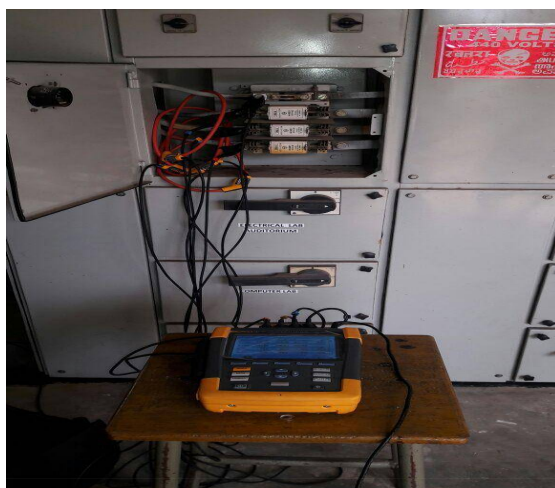
Fig.3.connection diagram of fluke 435-II with HT/LT side of the distribution transformer
